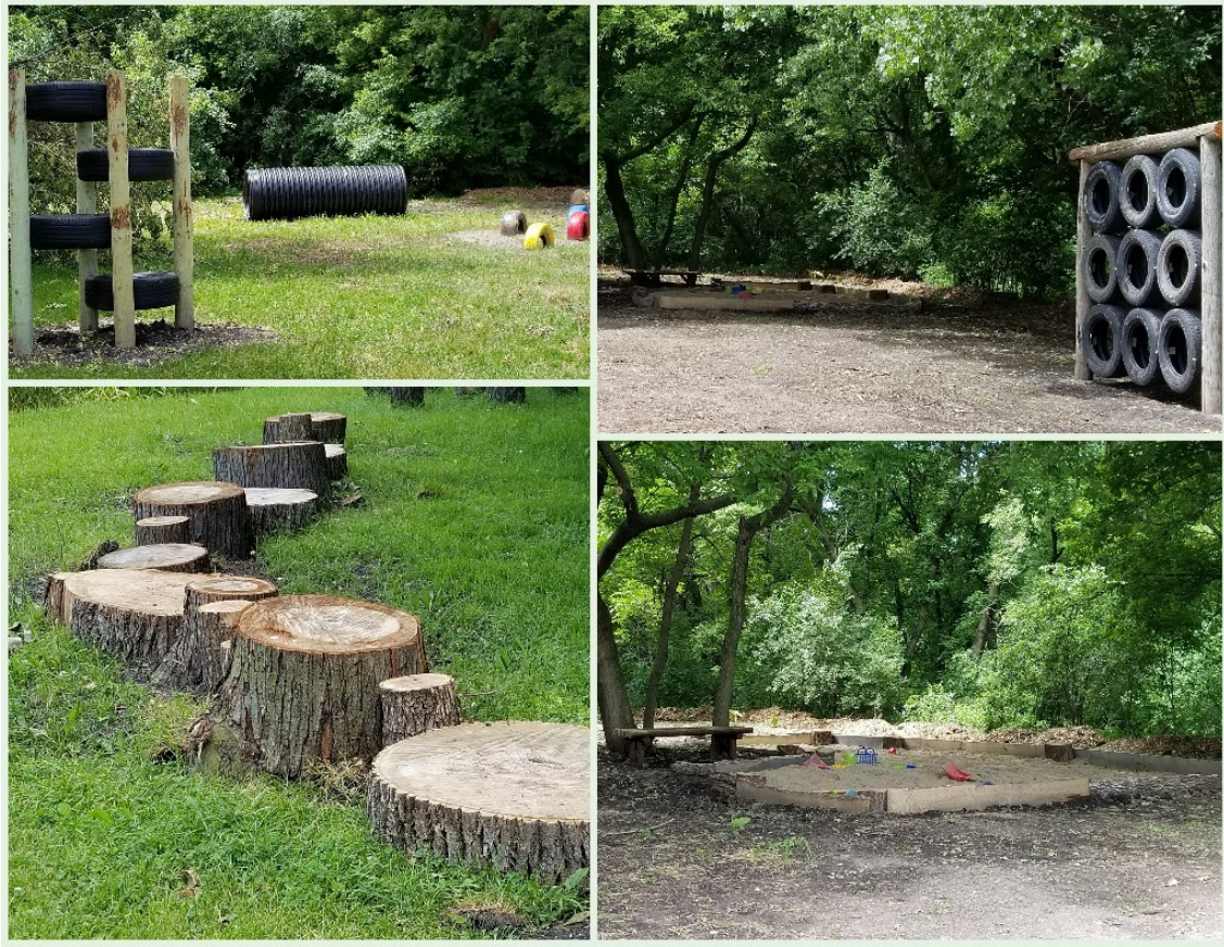
The new Adventure Park being constructed at the southern end of Lake Eagle Park
